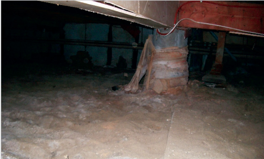
Figure 1 Crawl space before remediation
